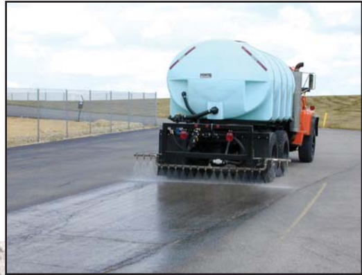
Dust Control Unit
